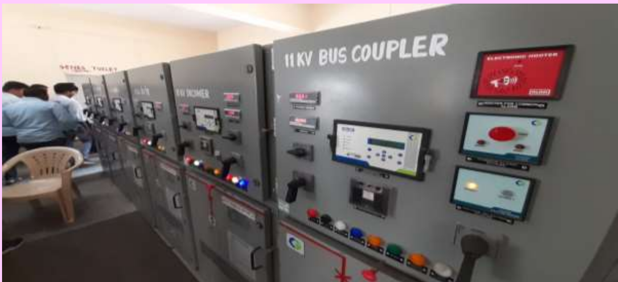
INDUSTRIAL VISIT NO-1 AT 33/11KV SHAHADA URBAN SUBSTAION AND 33/11KV GIS
