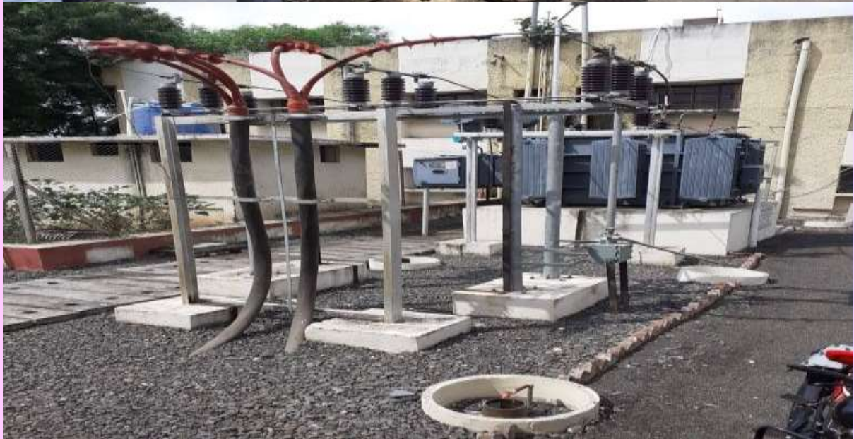
INDUSTRIAL VISIT NO-1 AT 33/11KV SHAHADA URBAN SUBSTAION AND 33/11KV GIS
